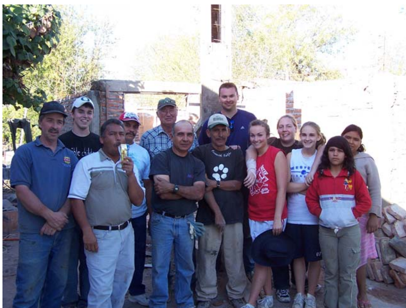
Nehemiah's wall builders have nothing on this smiling group of laborers (both US and Mexican) who spent 15 days building a parsonage and encouraging lives in northwestern Mexico.
