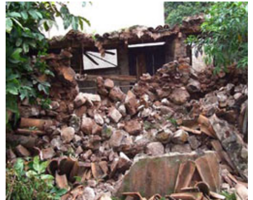
Rubble from Bukavu 6.0 earthquake
