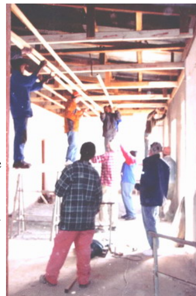
Bob Kauffman, Zion Mennonite, right foreground, directs building of frames for church lighting.
